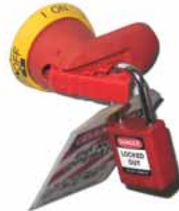
Figure 1: Lockout/Tagout on the Main Electrical Enclosure
