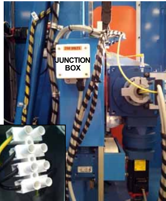
Figure 2: Junction Box in the Stroke/Elevation Chamber (on newer saws)
